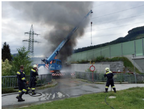
Taking into account all surrounding aspects can avoid damage, accidents and catastrophes.
